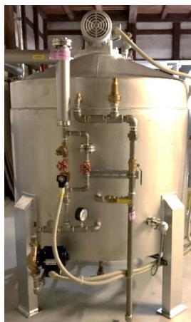
Side: Piping Part
