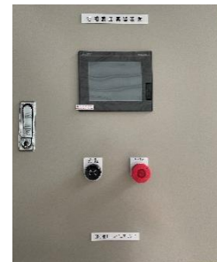
Touch panel control cabinet
